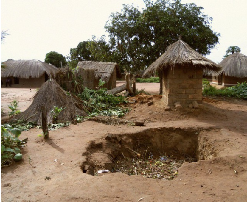
The thatched roof on the ground is where an outhouse just collapsed into its pit.
