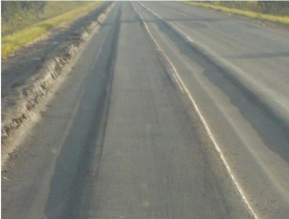
Heavy trucks make ruts in the hot asphalt.
